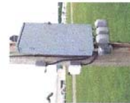
A typical electric hookup - multiple outlets per pole - all 30 amp receptacles - and 2 water faucets on each pole
